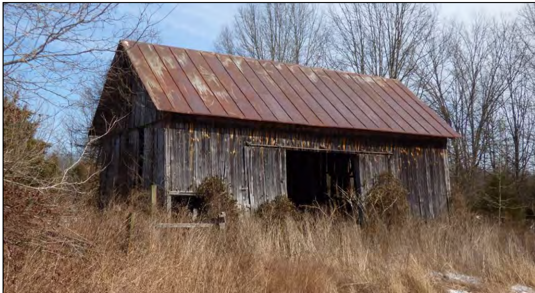
Photo 2: At Top, View of Stock Barn and Pumthouse Looking Northeast and, at Bottom, Southwest Oblique of Three-Bay, Multi-Purpose Barn (030-5540).
