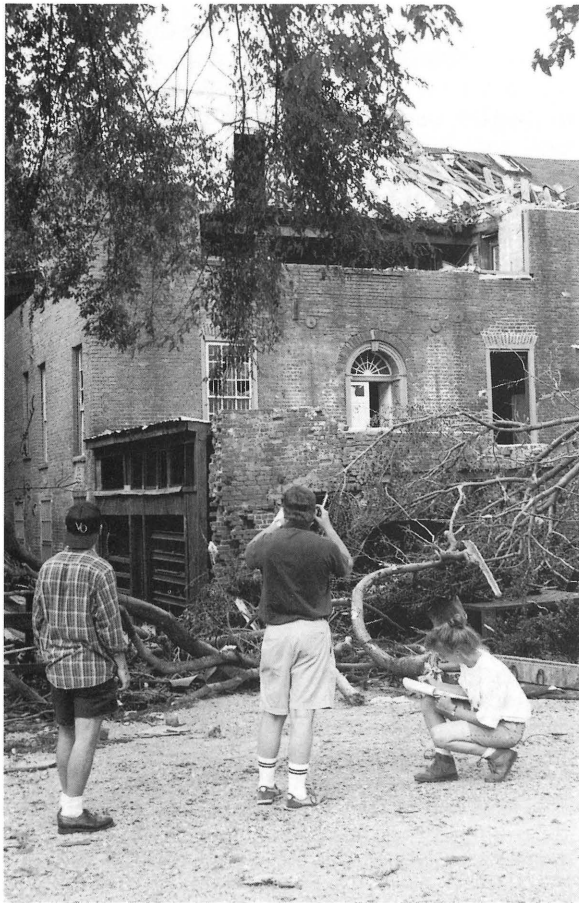
John Orrick, David Edwards and Elizabeth Lipford of the Department record the damage to the Appomattox Iron Works, a prominent Petersburg landmark.
