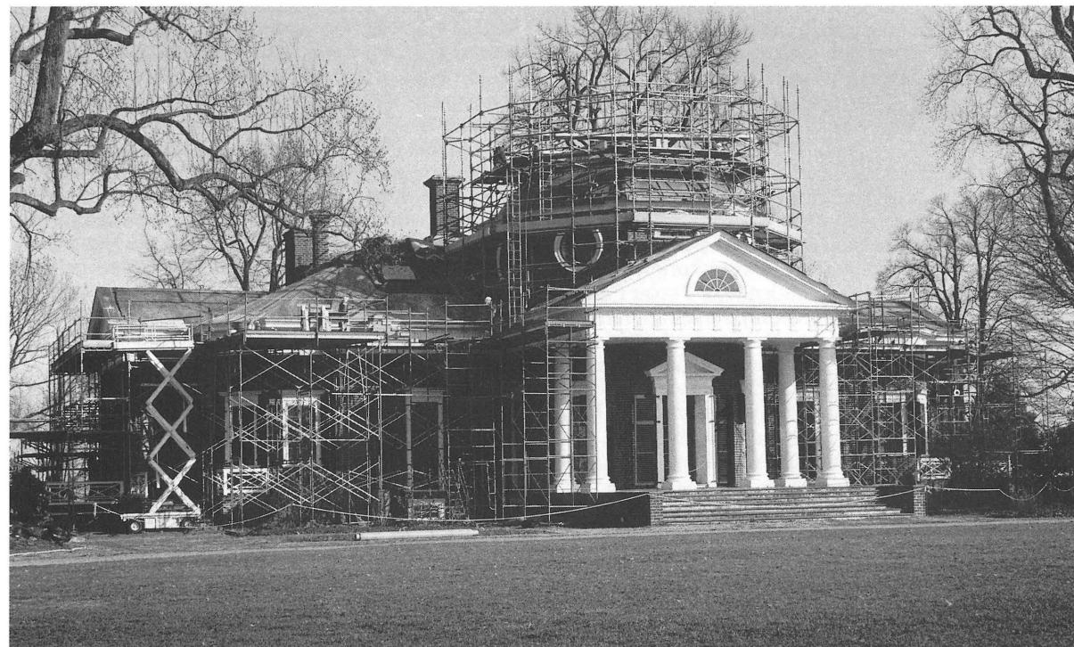
Monticello. Though somewhat foreign to most visitors' eyes, the scaffold-clad west front at Monticello would certainly have been familiar to Jefferson. Construction work of one sort or another was a constant during his lifetime. Courtesy of the Thomas Jefferson Memorial Foundation.
