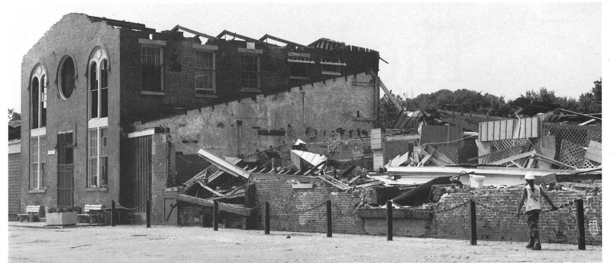
Petersburg South Side Railway Depot. The owners have rescued the antebellum roof trusses, removed debris and protected the standing sections of the building with temporary roofing. They are planning to rebuild.
