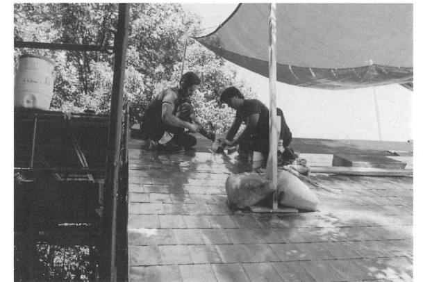
Replicas of Jefferson's tinplates, fabricated of terne-coated stainless steel, have now been installed over a watertight layer of neoprene on several of the pavilions and the student dormitories. Workers were careful to preserve Jefferson's original tinplates, discovered during restoration, under the new coverings. Courtesy of the University of Virginia, Facilities Management.
