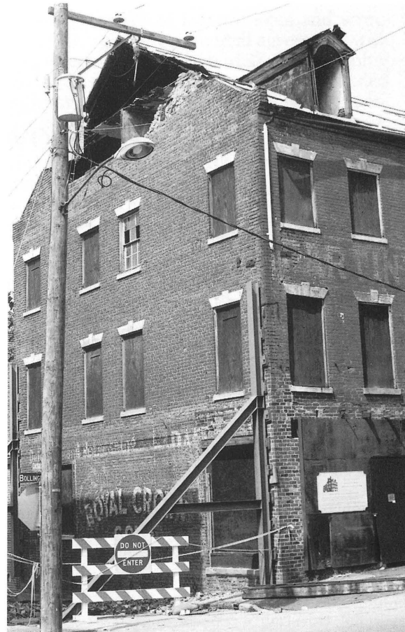
The Nathaniel Friend House, a registered Virginia landmark, sustained considerable damage to its walls and brick gables.
